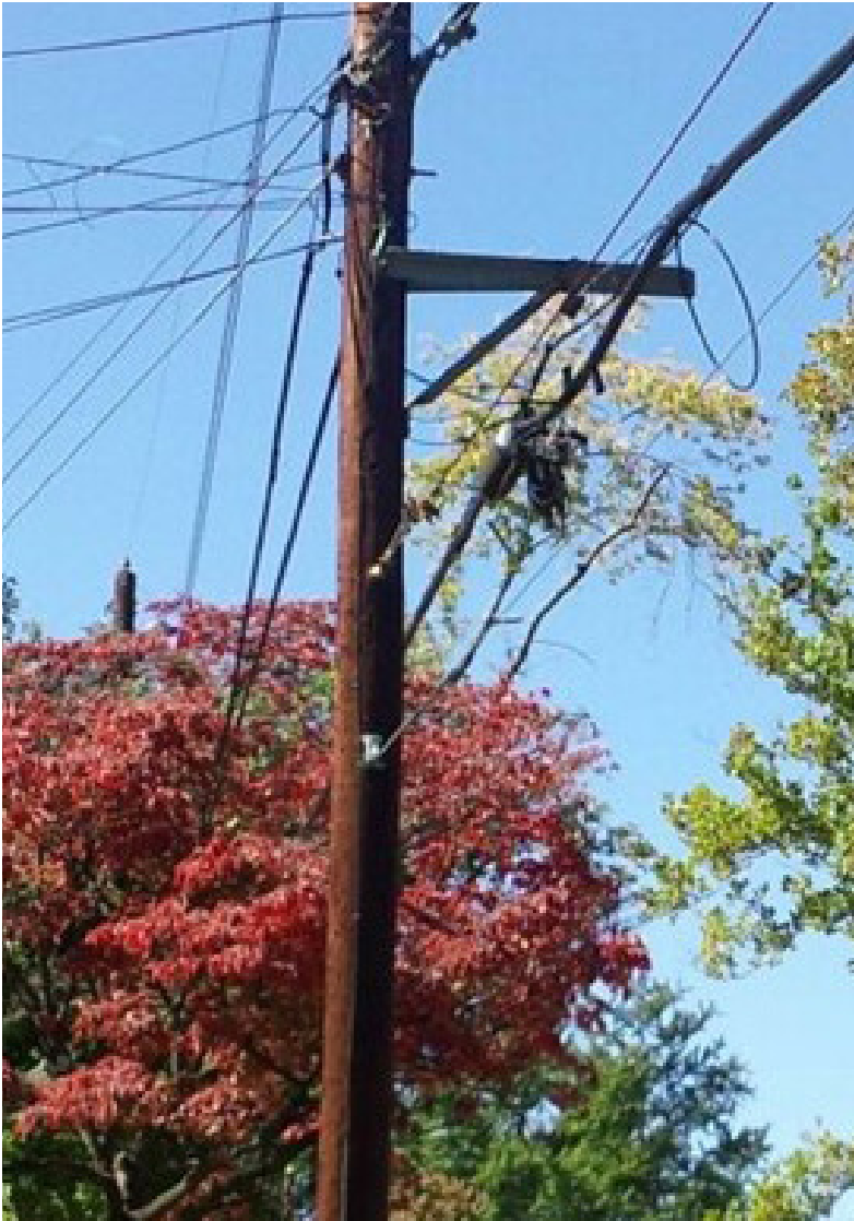
Figure 12: Example of extension arm on pole, enabling horizontal expansion of capacity
